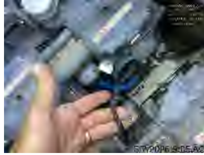
Cable spliced together then taped
